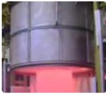
Bell Type Furnace
